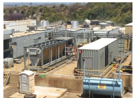
Power from engine waste heat, DOD/Guantanamo Bay, Cuba. Photo Courtesy Gulf Coast Clean Energy
