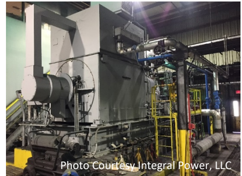
Photo Courtesy Integral Power, LLC It may not be pretty – but this turbine-generator set delivers 5 MW and offsets 159,000 ton/yr of CO2.
