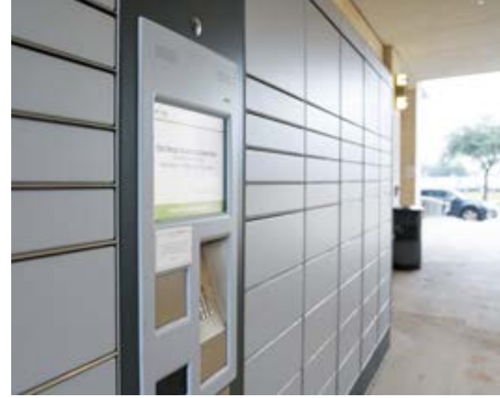
Package lockers were installed in all residential areas.
