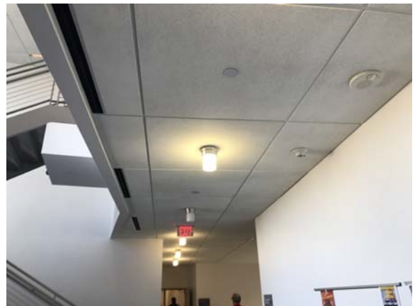
121039e 2/10/2022 Ceiling-mounted CFL lighting fixture Second floor corridor
