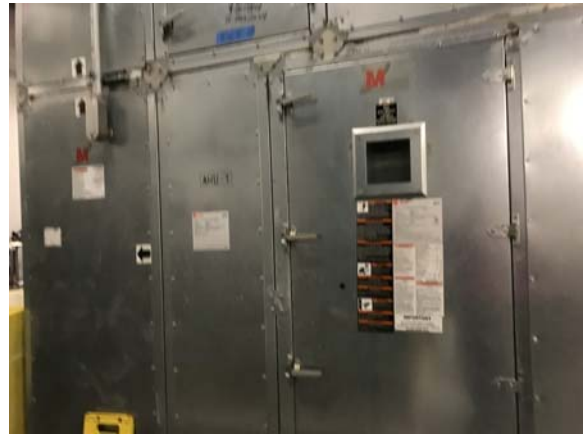
121050e 2/10/2022 Air handling unit AHU-2 Mechanical room 156
