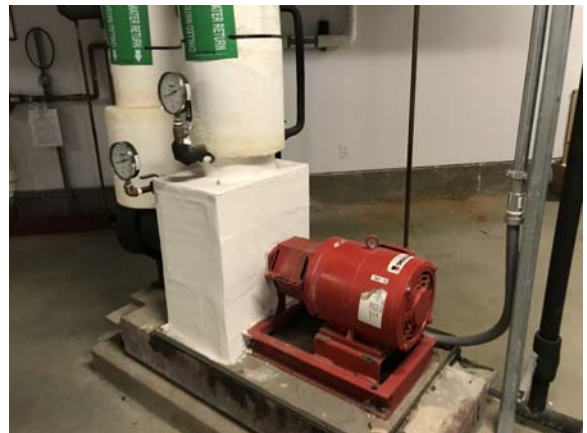
121015e 2/10/2022 Chilled water pump Penthouse
