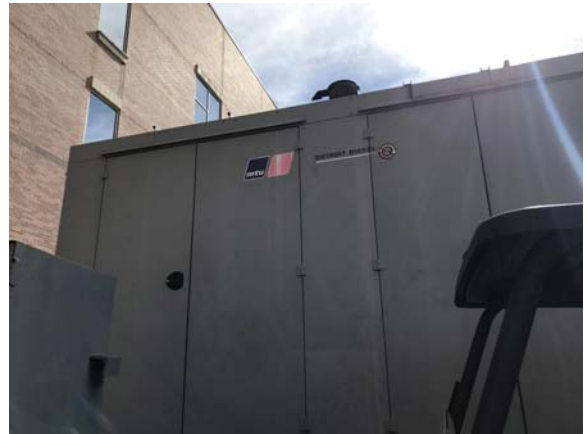
121056e 2/10/2022 Diesel-fired emergency generator Exterior courtyard
