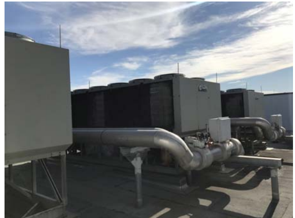
121002e 2/10/2022 Air-cooled packaged chillers Roof
