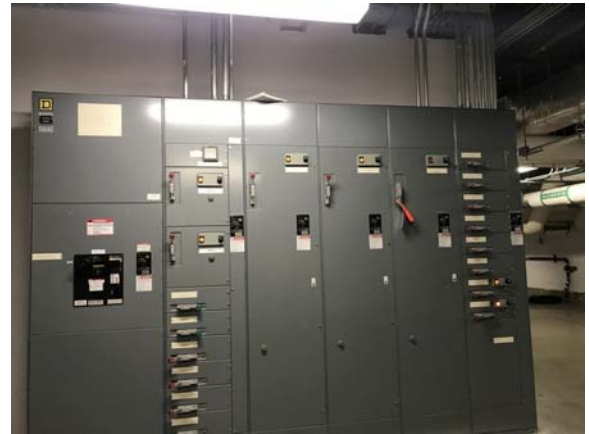
121010e 2/10/2022 Motor control center Penthouse
