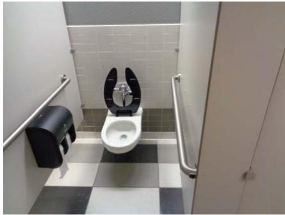
121037a 2/10/2022 Auto flush water closet Restroom
