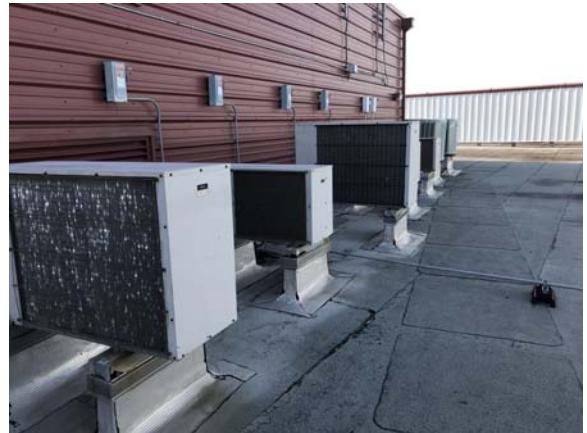
121008e 2/10/2022 Ductless split condensing units Roof
