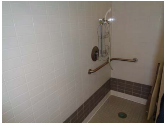
121040a 2/10/2022 Shower head and valve Restroom
