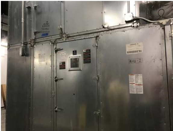
121049e 2/10/2022 Air handling unit AHU-1 Mechanical room 156
