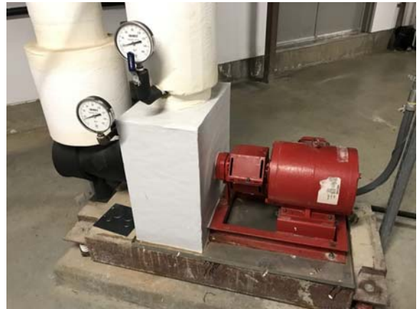
121019e 2/10/2022 Chilled water pump Penthouse
