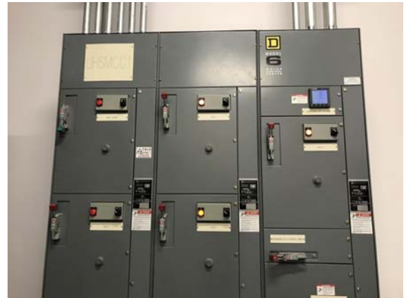
121047e 2/10/2022 Motor control center Main electrical room 154
