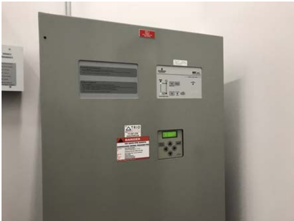
121057e 2/10/2022 Automatic transfer switch Main electrical room 154
