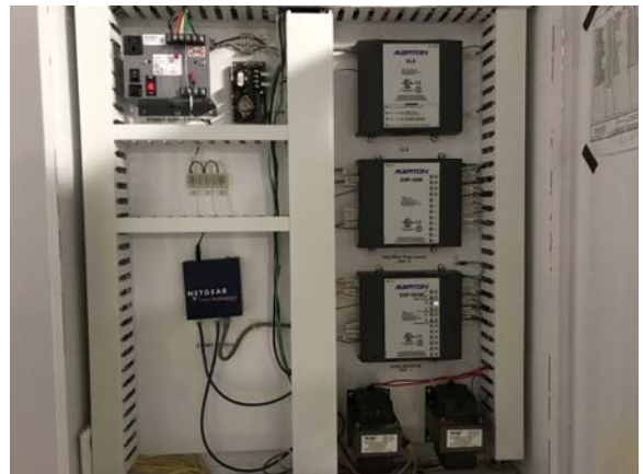
121024e 2/10/2022 HVAC field panel Penthouse
