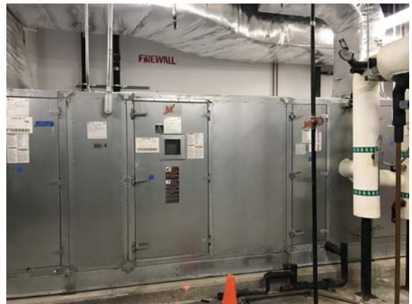
121036e 2/10/2022 Air handling unit AHU-4 Mechanical room 246
