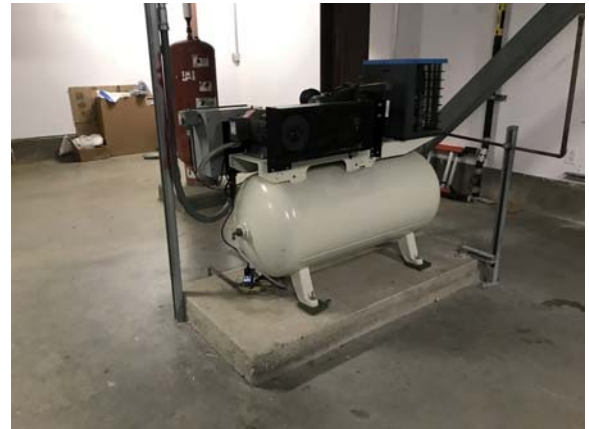
121011e 2/10/2022 Process air compressor Penthouse
