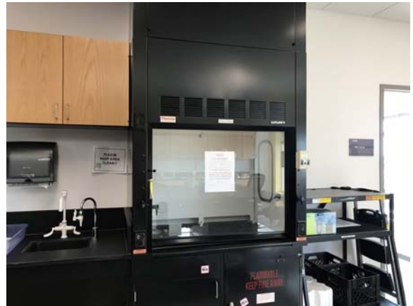
121028e 2/10/2022 Typical laboratory fume hood Laboratory 355
