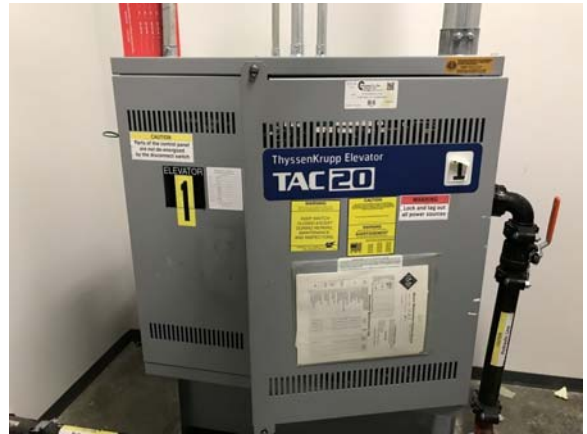
121043e 2/10/2022 Elevator 2 hydraulic controls Elevator mechanical room 158
