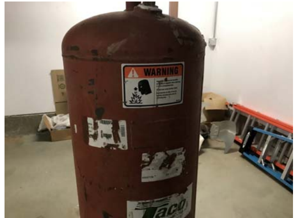
121013e 2/10/2022 Chilled water expansion tank Penthouse
