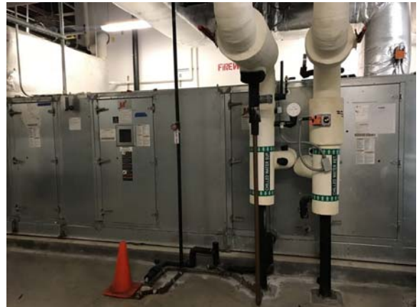
121025e 2/10/2022 Air handling unit AHU-6 Mechanical room 346
