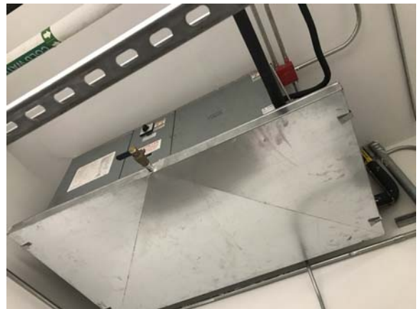
121045e 2/10/2022 Fan coil unit Main electrical room 154
