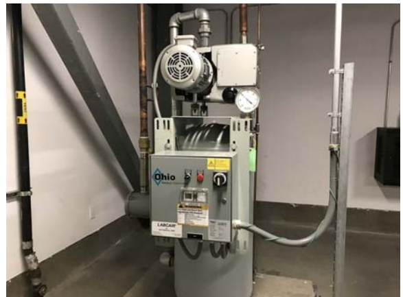
121009e 2/10/2022 Rotary vane vacuum pump system Penthouse
