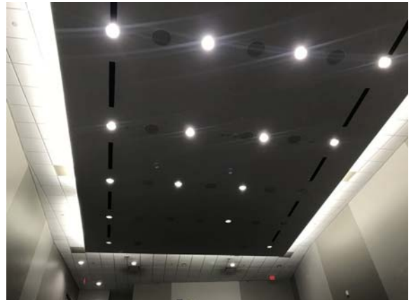
121041e 2/10/2022 Recessed can HID lighting fixtures Room 280
