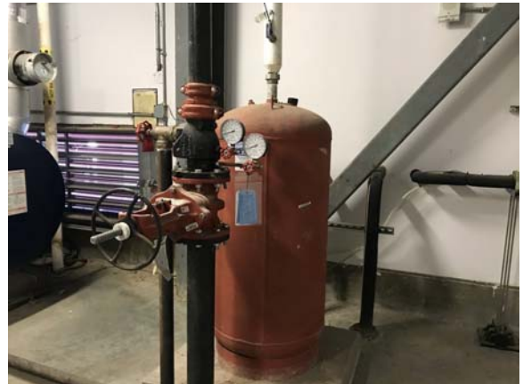
121023e 2/10/2022 Domestic hot water expansion tank Penthouse
