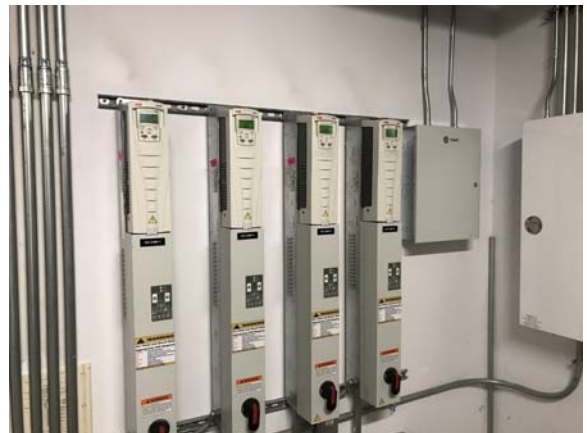
121018e 2/10/2022 VFDs for chilled water pumps Penthouse
