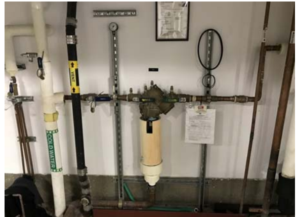
121017e 2/10/2022 Backflow preventer for makeup water Penthouse
