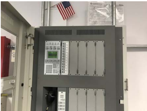
121059e 2/10/2022 Main fire alarm panel Room 174
