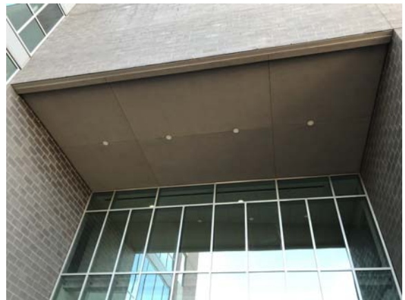
121060e 2/10/2022 Recessed can lighting fixtures Exterior soffit
