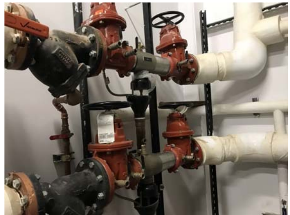
121054e 2/10/2022 Backflow preventers for water main Mechanical room 156
