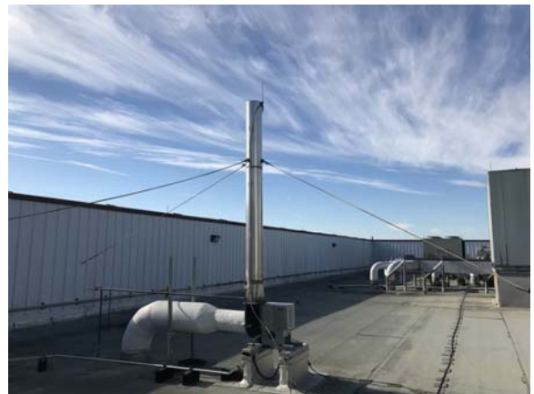
121006e 2/10/2022 Utility exhaust fan Roof
