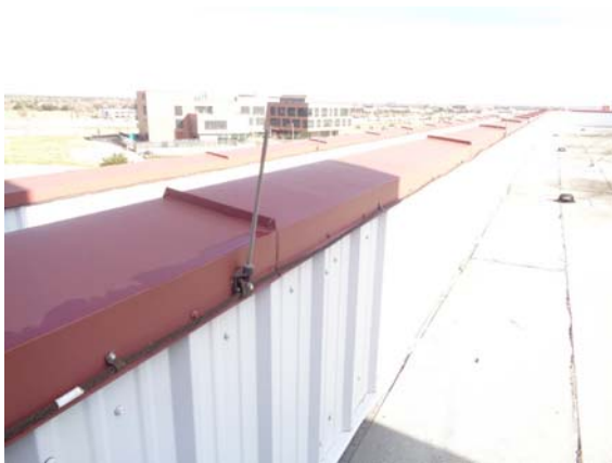
121045a 2/10/2022 Lightning protection system Main roof
