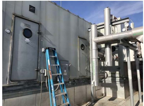
121004e 2/10/2022 Air handling unit EARU-2 Roof
