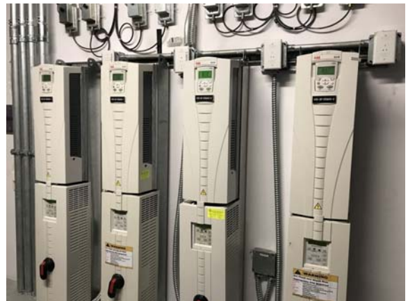
121021e 2/10/2022 VFDs for EARU supply fans and exhaust fans Penthouse
