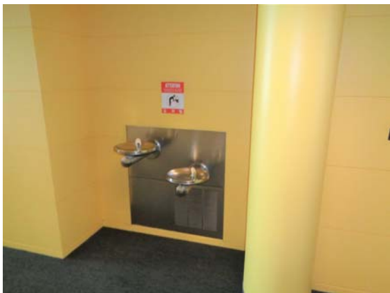
121036a 2/10/2022 Dual-level drinking fountains Corridors
