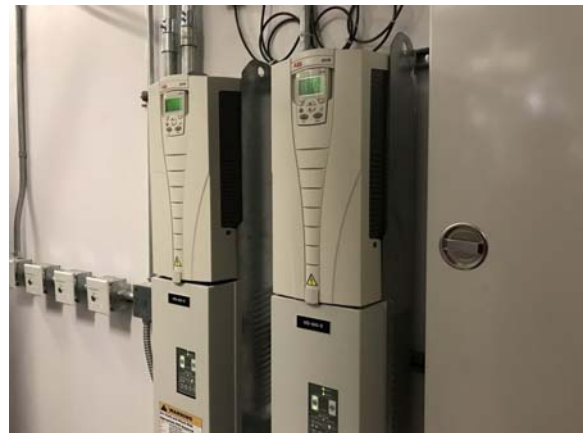
121027e 2/10/2022 VFDs for AHU-5 and AHU-6 Mechanical room 346
