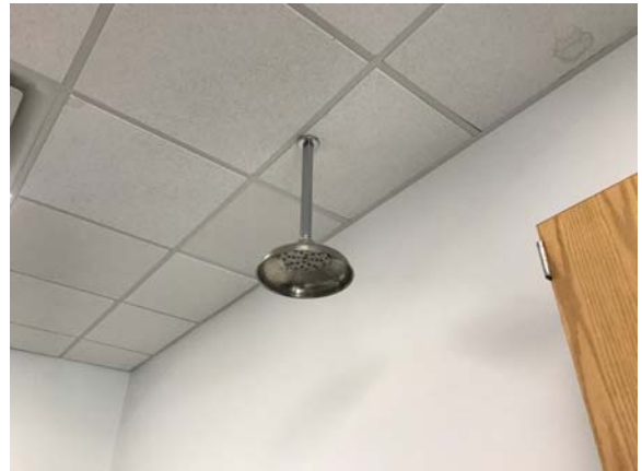
121029e 2/10/2022 Typical emergency shower Laboratory 355
