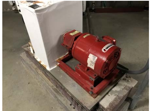
121016e 2/10/2022 Chilled water pump Penthouse
