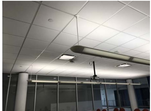
121040e 2/10/2022 Suspended T8 lighting fixture Room 247
