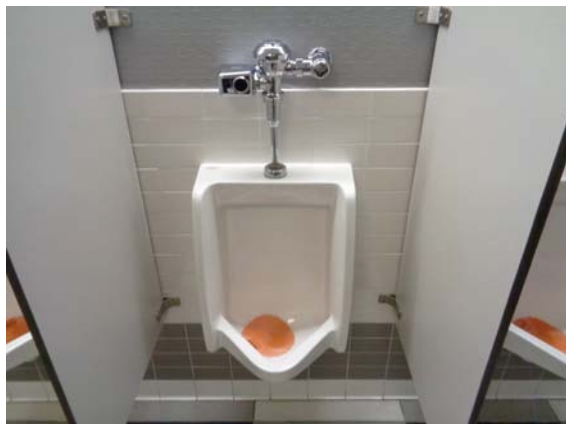
121039a 2/10/2022 Auto flush urinal Restroom
