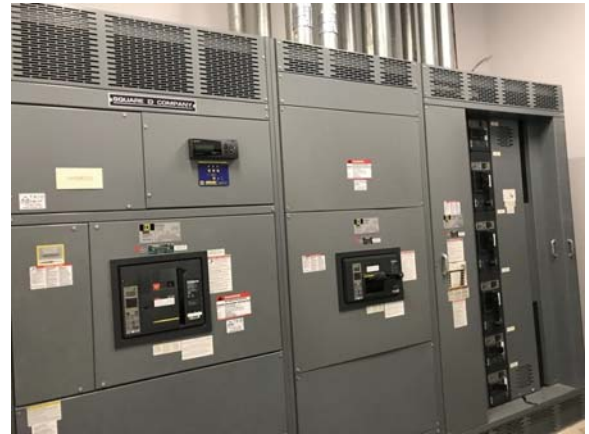
121046e 2/10/2022 Main switchboard Main electrical room 154
