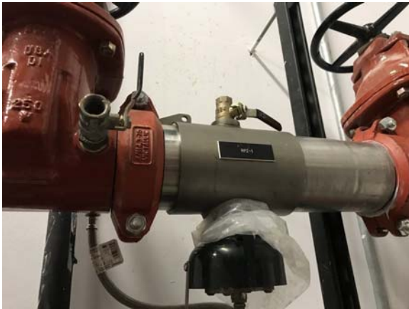
121055e 2/10/2022 Backflow preventer for fire suppression Mechanical room 156
