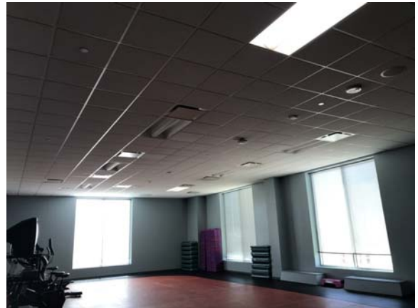
121058e 2/10/2022 Recessed CFL and T8 lighting fixtures Room 149
