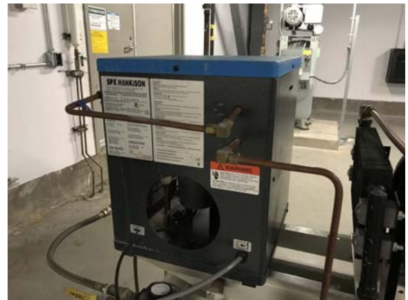
121012e 2/10/2022 Refrigerated air dryer Penthouse
