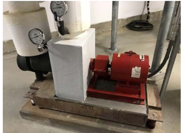
121020e 2/10/2022 Chilled water pump Penthouse
