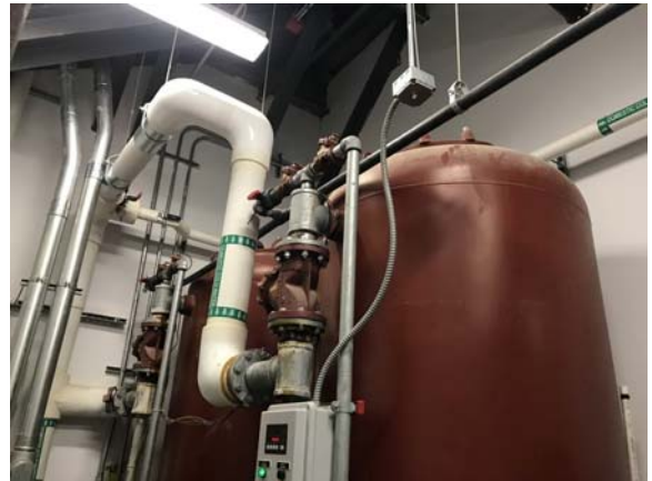
121052e 2/10/2022 Industrial water softener Mechanical room 156
