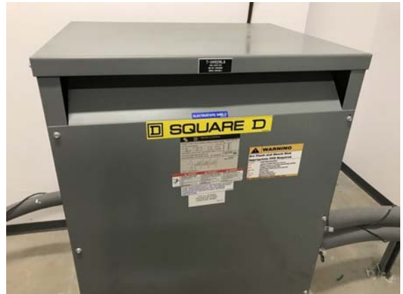
121038e 2/10/2022 Typical dry-type transformer Electrical room 256
