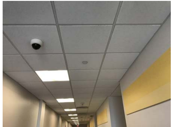
121031e 2/10/2022 Fire suppression sprinkling device Third floor corridor
