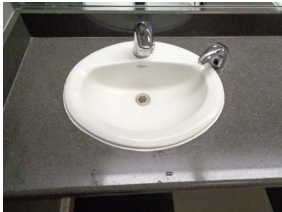
121038a 2/10/2022 Auto sensor vanity Restroom
