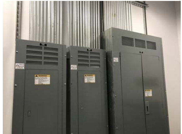
121037e 2/10/2022 Local panelboards Electrical room 256
