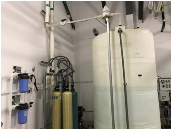
121051e 2/10/2022 RO system and storage tank Mechanical room 156
