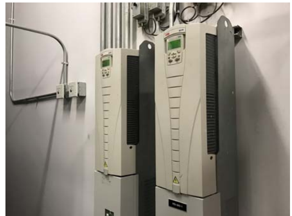
121048e 2/10/2022 VFDs for AHU-1 and AHU-2 Mechanical room 156
