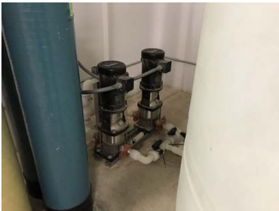
121053e 2/10/2022 RO pumps Mechanical room 156
