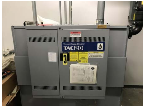
121044e 2/10/2022 Elevator 1 hydraulic controls Elevator mechanical room 158
