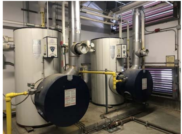
121022e 2/10/2022 Commercial gas-fired water heaters Penthouse
