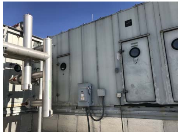
121003e 2/10/2022 Air handling unit EARU-1 Roof
