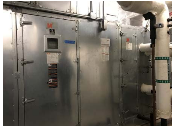
121026e 2/10/2022 Air handling unit AHU-5 Mechanical room 346
