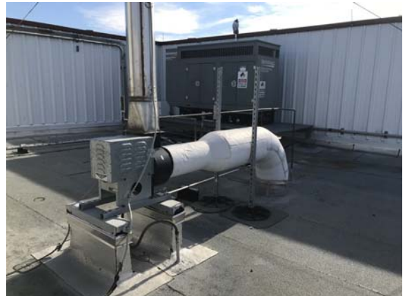
121005e 2/10/2022 Utility exhaust fan Roof
