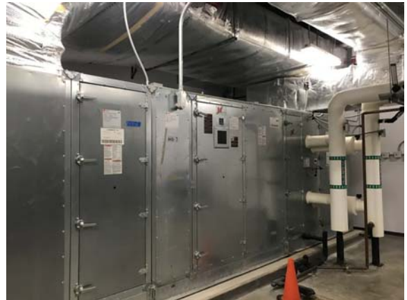
121035e 2/10/2022 Air handling unit AHU-3 Mechanical room 246
