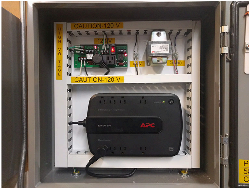
FIGURE B: HIGH VOLTAGE PANEL
