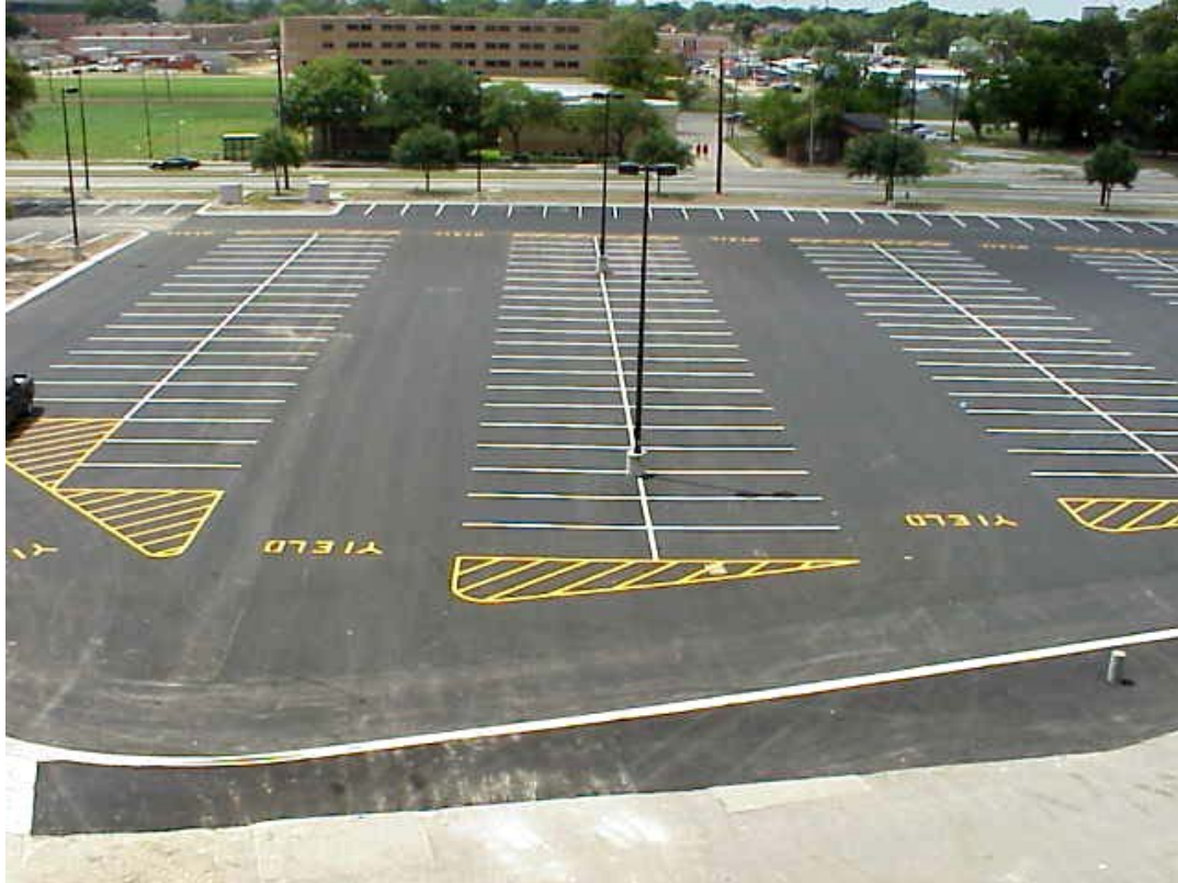
FIGURE 1.1 OVERVIEW OF PARKING LOT AND LIGHTING
